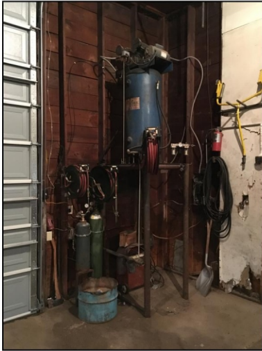
SMC 220V Air Compressor w/All Attachments. Will be sold in place.
